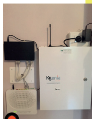
Ksenia Security control panel lares 4.0
